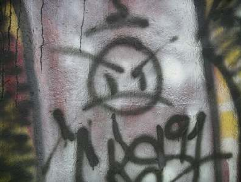
Smiley Face graffiti; located under the Ford Avenue Bridge (East bank), May 15, 2010.
