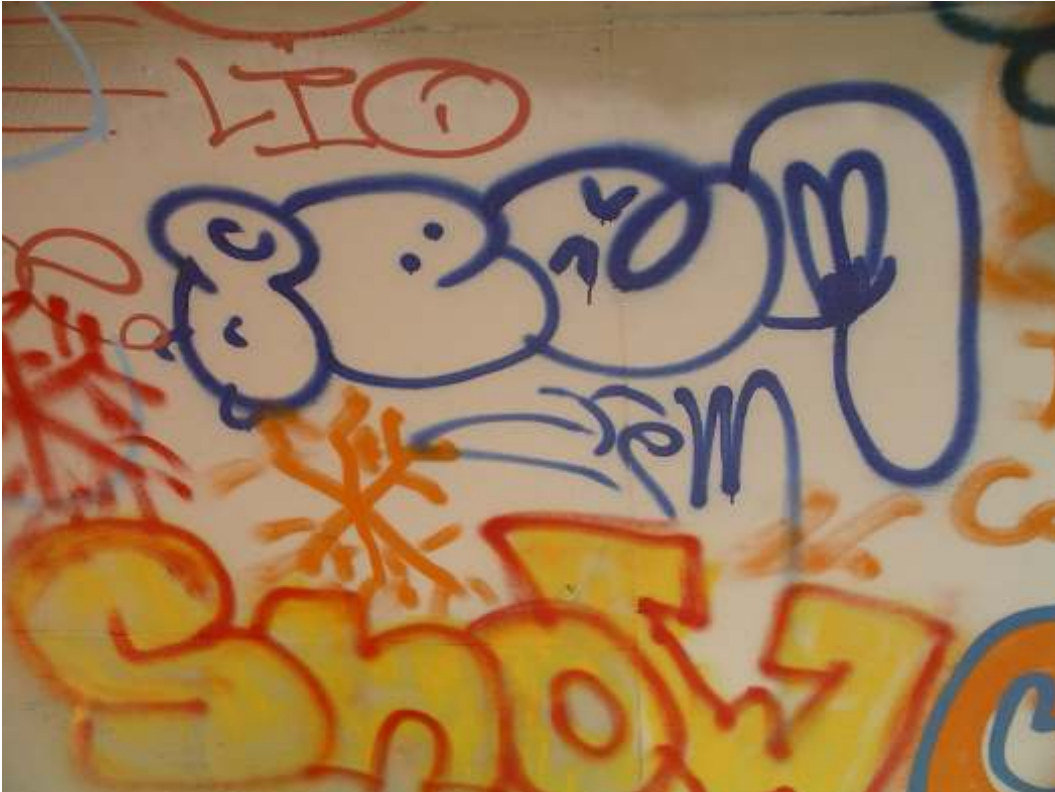
Smiley Face graffiti; located under the Franklin Avenue Bridge approach span (East bank), March 17, 2010.
